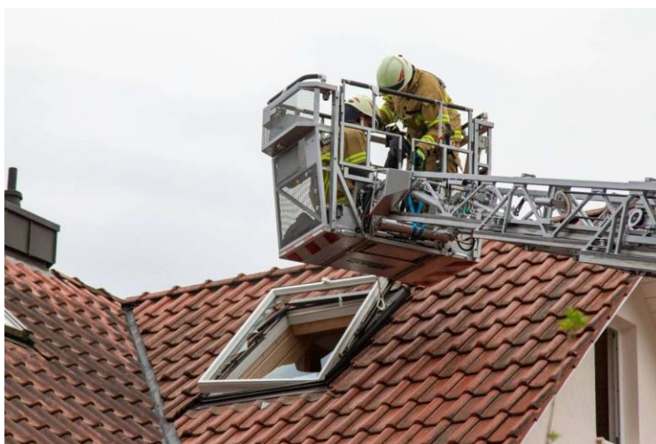
Figure 9 – Damage to window during incident [16].
