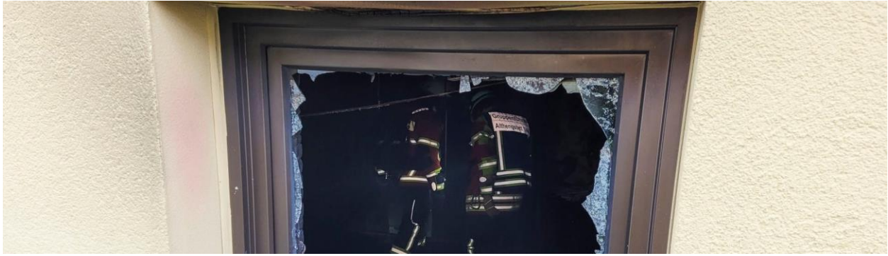
Figure 15 – Window damaged by explosion [23].
