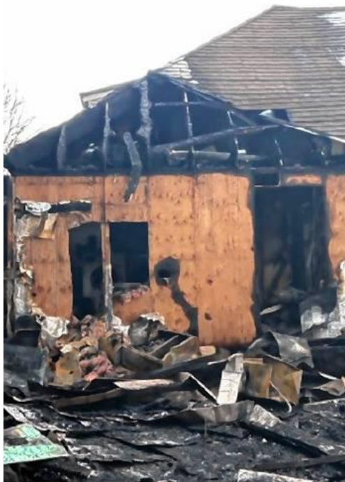
Figure 18 – Fire damage to property following lithium ion battery thermal runaway [24].
