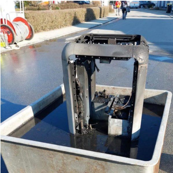
Figure 11 – ESS unit condition after firefighting operations [11].
