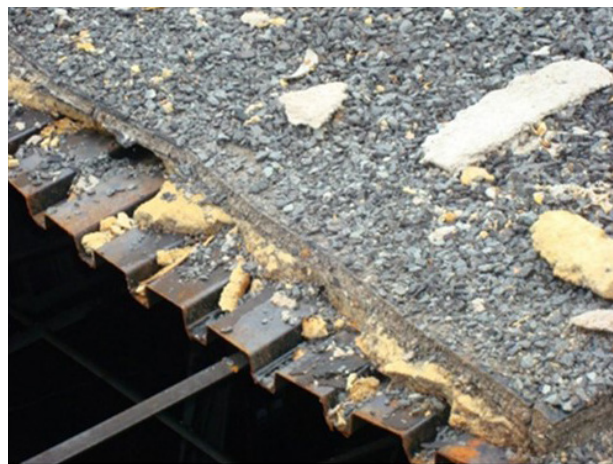
Photo 1. Construction of flat metal roof covered with asphalt foam insulation, and gravel. Chain saws were initially used to open the roof for vertical ventilation but would not cut through the metal deck. A circular saw with metal cutting blade had to be used.
