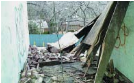
Right: Structural failure and collapse contributed to 43 percent of fireground deaths between 1999 and 2004.
